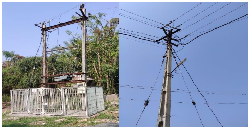
Figure 32: Electrical Facilities in Bhutsad
