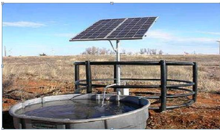
Figure 57: Solar Based Water Pump
